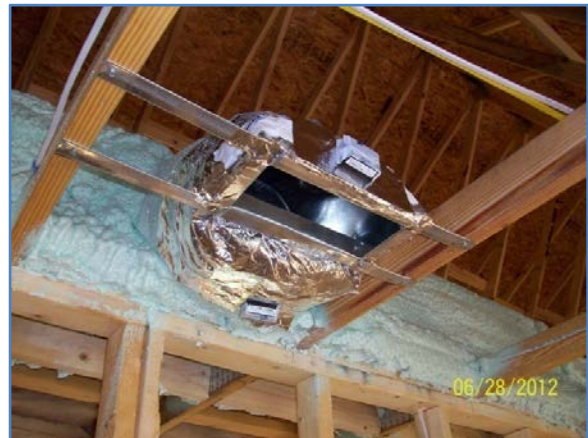
Figure 20. Supply register boot near an interior wall
