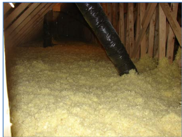
Figure 16. Ducts deeply buried in attic insulation
