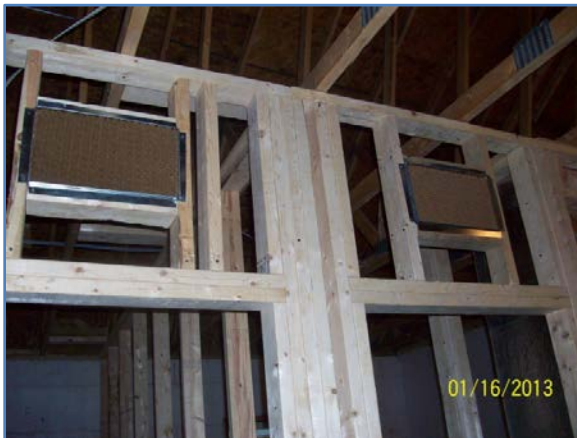
Figure 19. Bedroom transfer grilles
