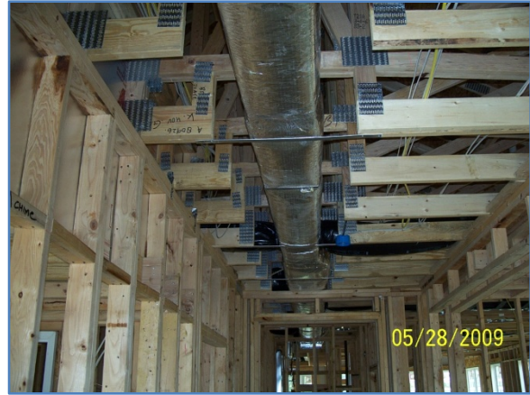
Figure 13. Truss chase with supply trunk
