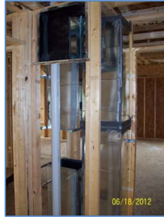
Figure 18. Central duct chase and return
