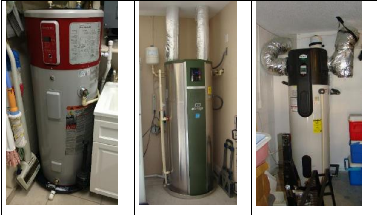
Figure 5. Heat pump water heater configurations: Left, interior GE unit in utility room at Site 13; center, ducted AirGenerate unit at Site 5; right, ducted A.O. Smith unit at Site 26
