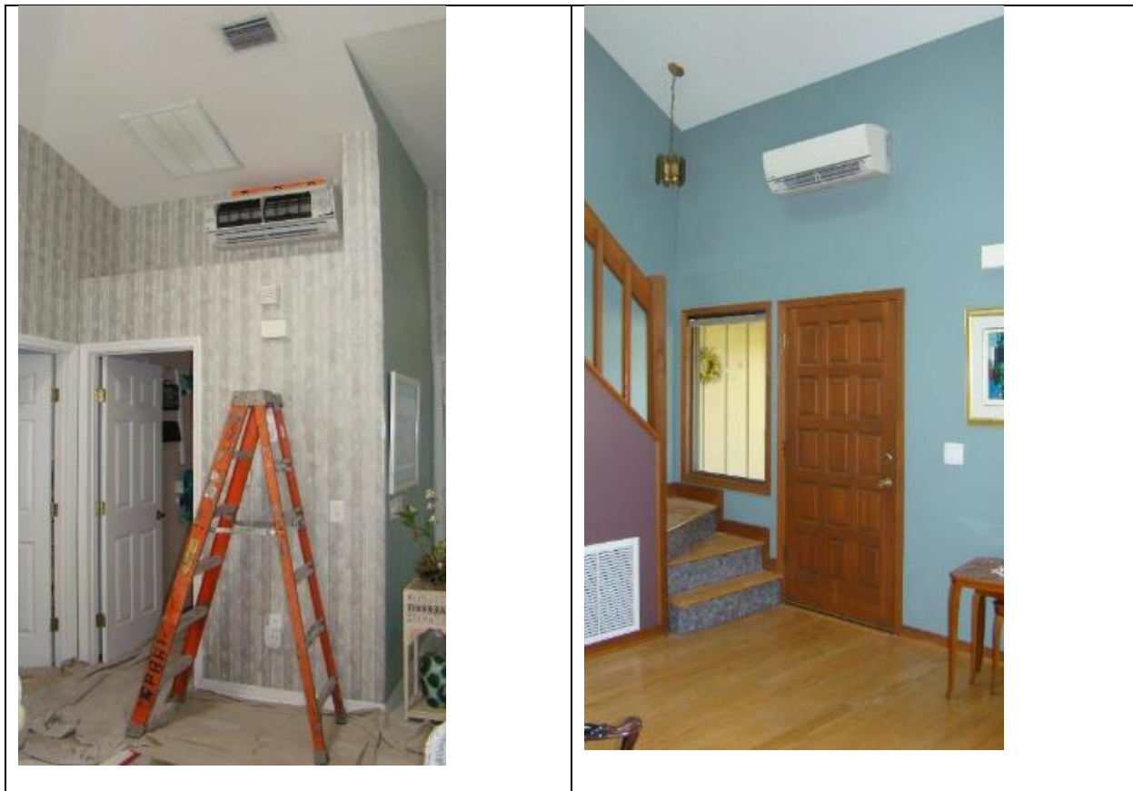
Figure 1. Wall-mounted mini-split heat pump fan coil at Site 3 and Site 24
