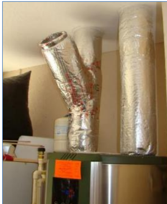
Figure 12. Y-type ducting arrangement at Site 5 allowing cold exhaust air to be diverted from the conditioned living environment
