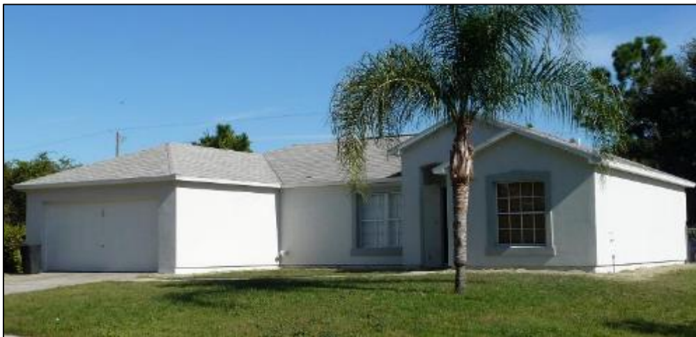
Figure 14. Site 54 attachment of 2-inch polystyrene insulation (top left), final textured coat application (top right), completed exterior insulation finish system retrofit (bottom)
