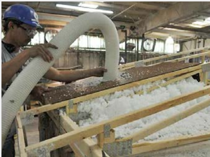
Blown fiberglass is dense packed into the roof eaves using a removable baffle
