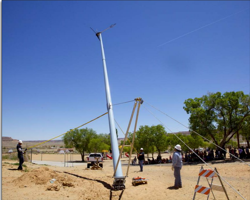
Photo from Westwind Solar Electric, Inc., NREL 18820
