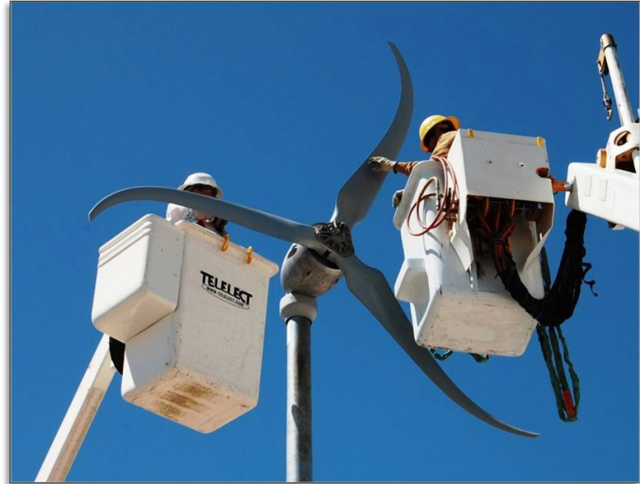
Photo from Chris Brooks, NREL 16743
