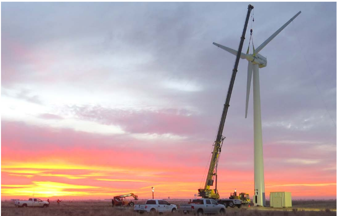
Sandia National Laboratories' successful remount of a turbine rotor at the Scaled Wind Farm Technology Facility (shown here) marked the beginning of several research projects at the facility on behalf of DOE's Atmosphere to Electrons initiative. Photo from Josh Bryant, Westergaard Solutions
