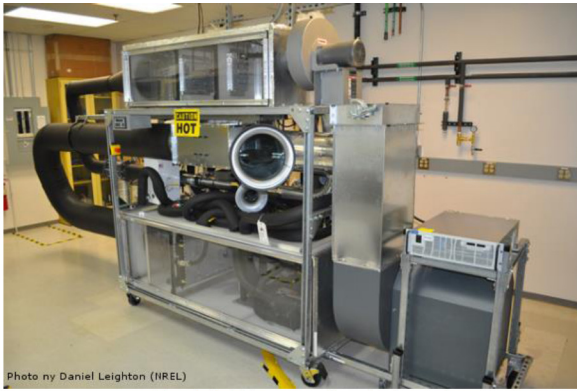
Figure 3. NREL's combined fluid loop test bench thermal management system apparatus
