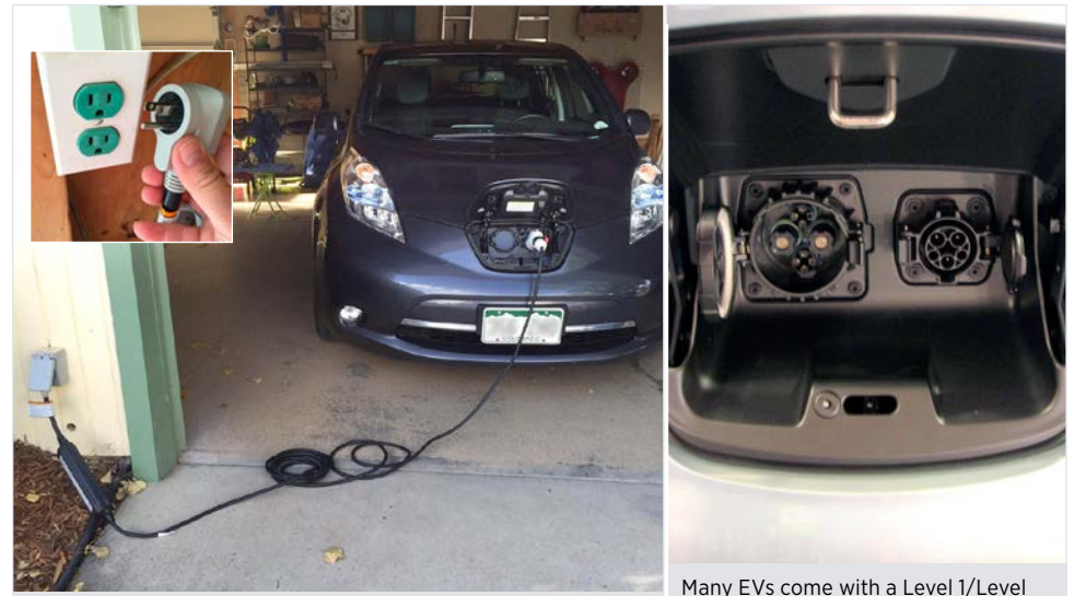
A “Level 1” cordset can be plugged in to a typical dedicated, 110-volt household outlet. Photos by Erik Nelsen, NREL 34794 (above) and 37587 (inset)
