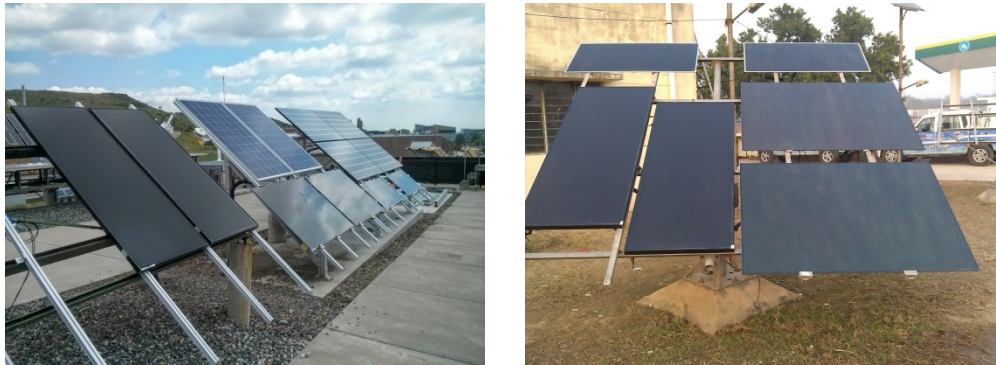
Figure 1. Thin film modules deployed at NREL (left) and NISE (right)
