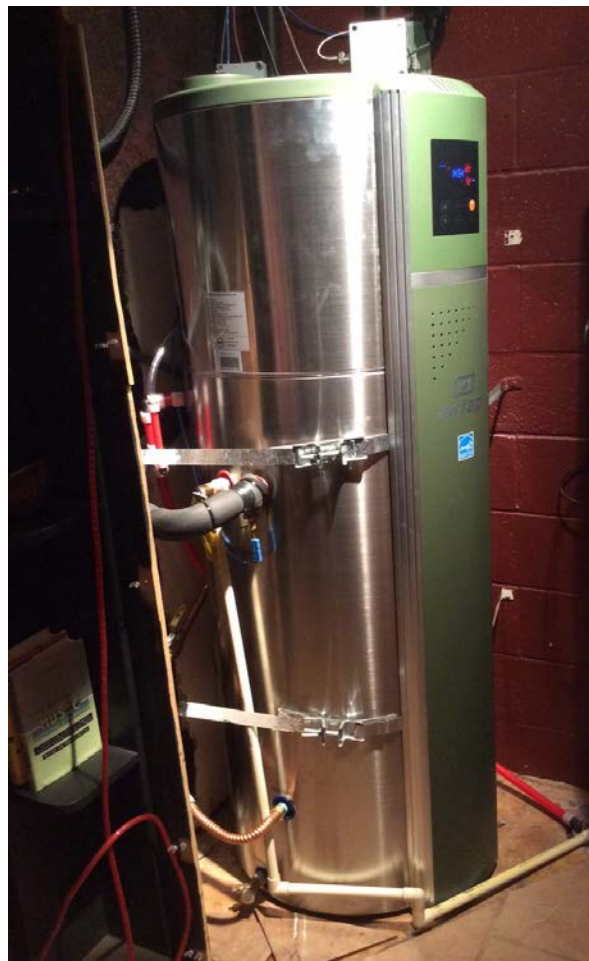
Figure 11. Installed HPWH at Site 1
