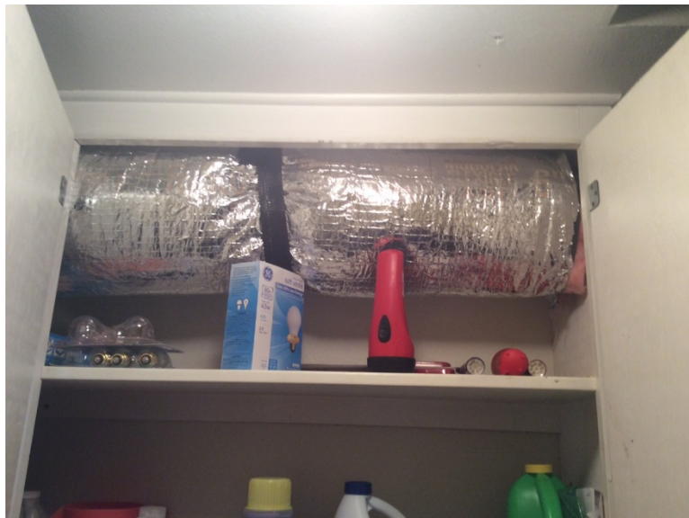
Figure 12. Site 2 ducting run to outdoors
