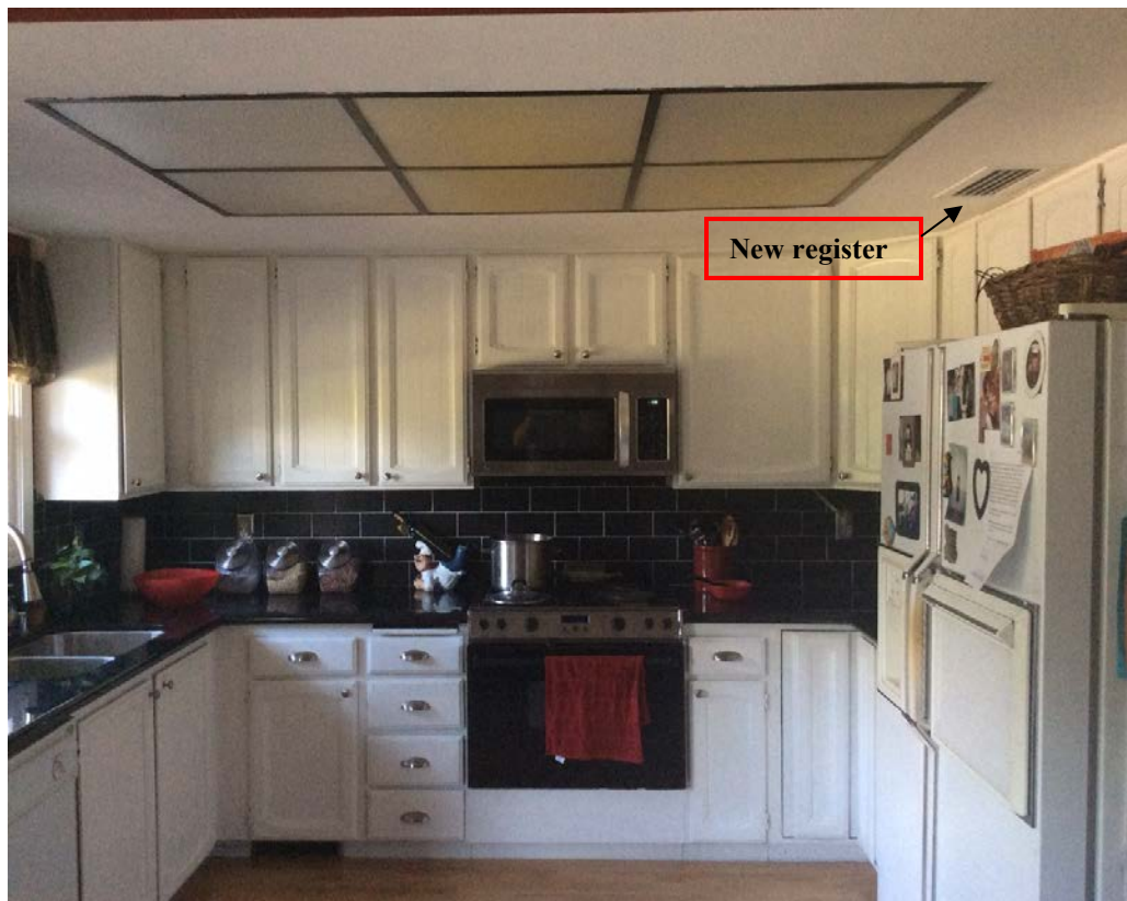
Figure 13. Site 2, HPWH evaporator leaving air discharge to kitchen
