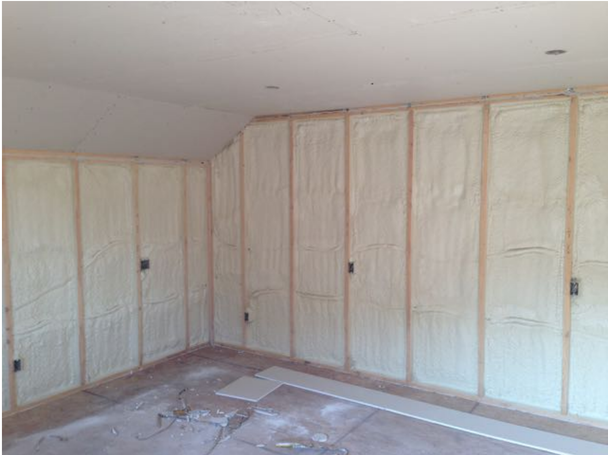
Figure 20. Amaris Custom Homes: Advanced frame wall with spray foam insulation of the Mound, Minnesota, project
