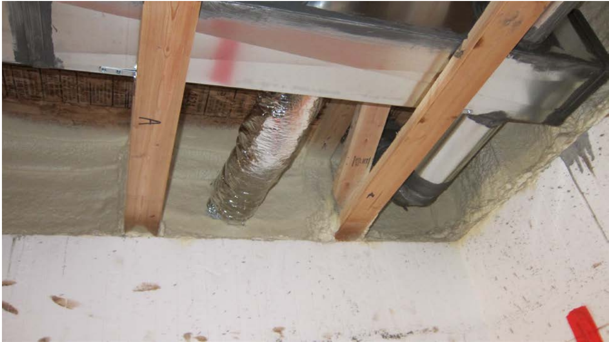
Figure 32. Urban Homeworks: ICF foundation, closed-cell spray foam at rim joist, and sealed ductwork located within the thermal enclosure of the North Minneapolis, Minnesota, project
