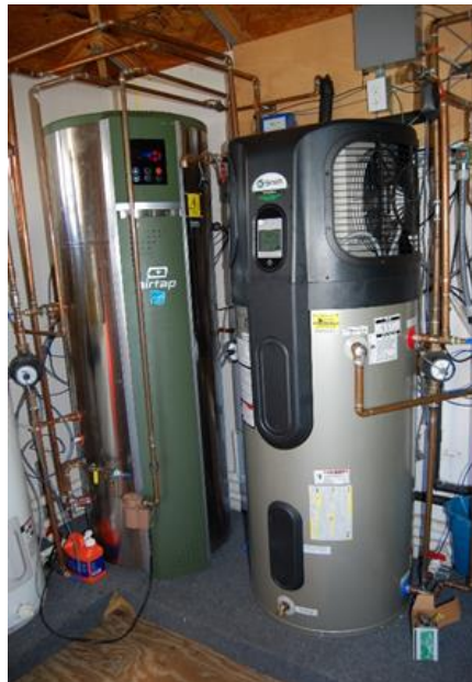
Figure 3. Two heat pump water heaters of large and medium storage capacity (80 and 60 gallons) High-efficiency natural gas: AOSmith HYB 90N
