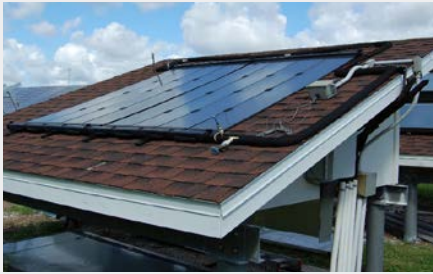
Figure 4. The solar polymer system with lightweight collectors (27 lbs. each) has a lower installed cost potential than standard solar systems. It also demonstrated an average electric reduction of 36%, partly impaired by long length (72 ft. one-way) circulation lines. The polymer open-loop system is also freeze tolerant.
