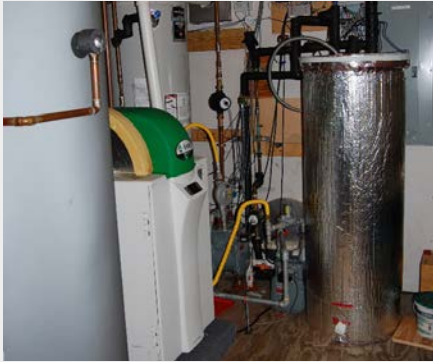
Figure 3. Hybrid gas heater (pictured left) with small hot water storage—relative to tankless—reduces hot water delay to point of use, promoting water conservation with a relative high efficiency (COP 0.74).
