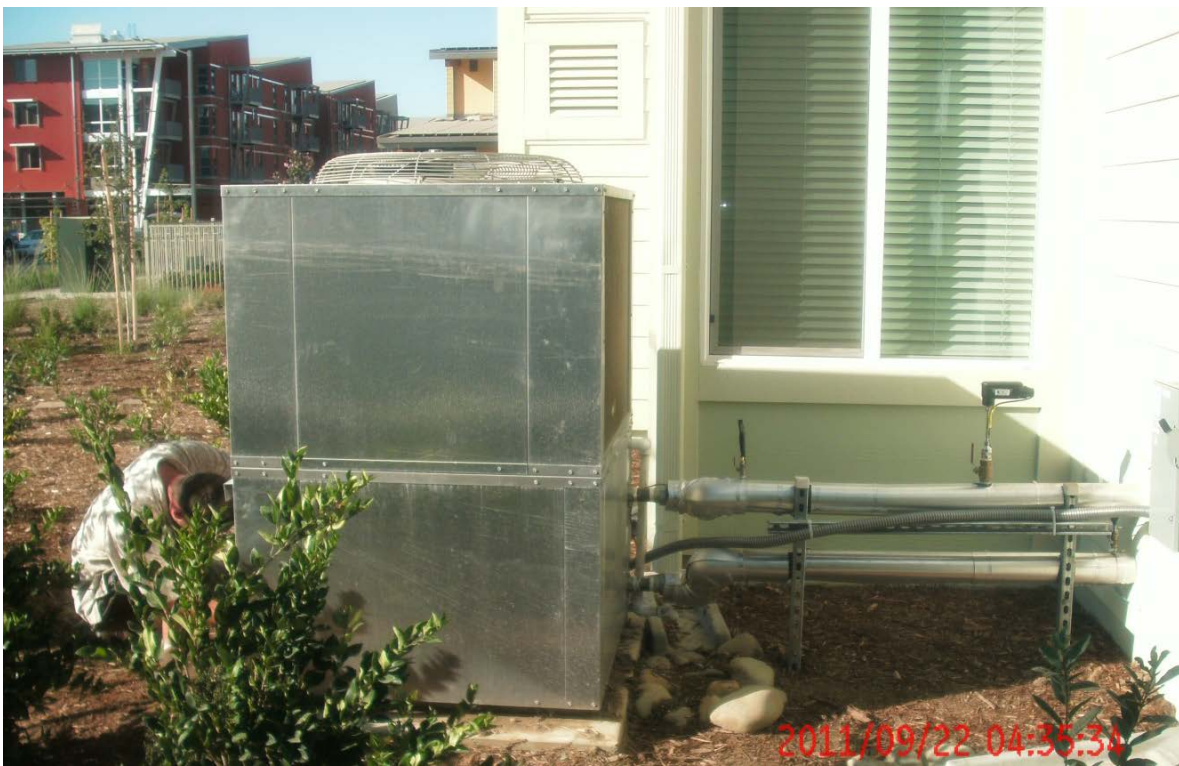
Figure 4. Monitored HPWH outdoor unit
