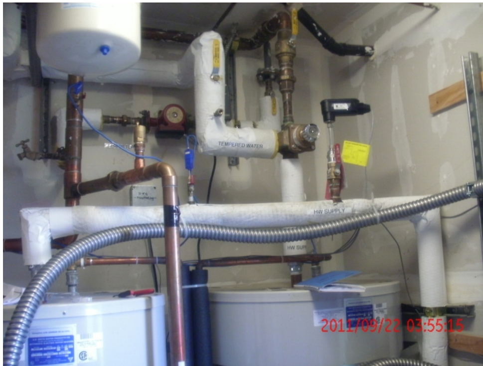
Figure 5. Electric resistance storage tanks with capacities of 120 gal with piping and monitoring sensors
