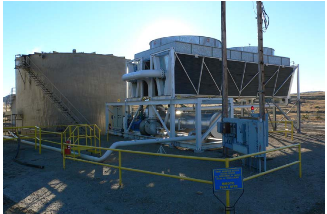
250 kW geothermal coproduction demonstration system at Rocky Mountain Oilfield Testing Center
