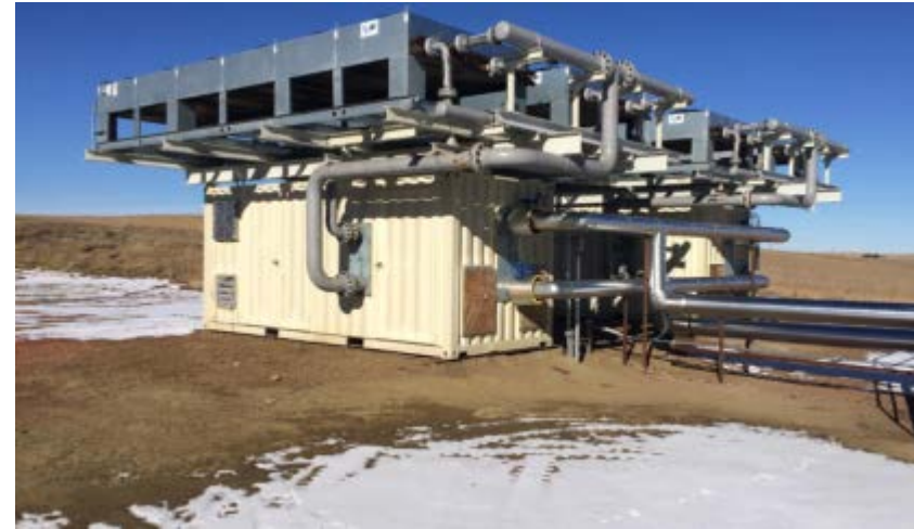
Power Generation Units
