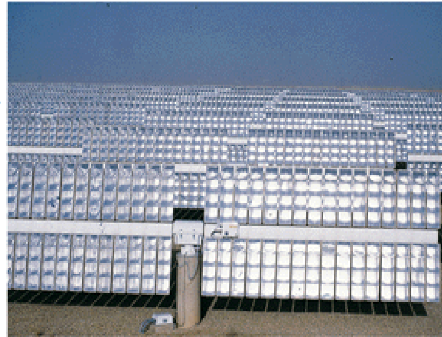
Photograph of the SolERAS site. See also: Bowen, Proc PLEA Conf. , 1985.
