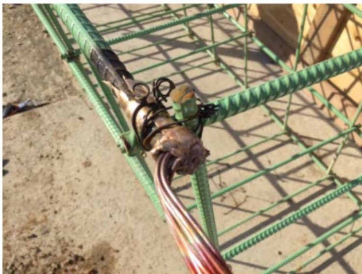
Figure 7. New grounding required for vehicle fueling
