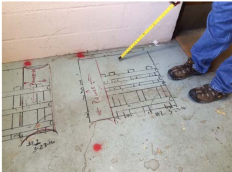
Figure 8. Review of below-grade images required to locate rebar for station fueling pad
