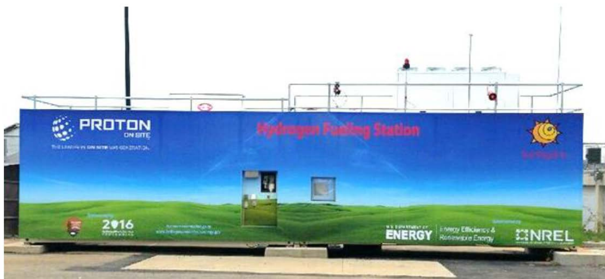
Figure 4. Photo of the installed hydrogen fueling station at the Brentwood site
