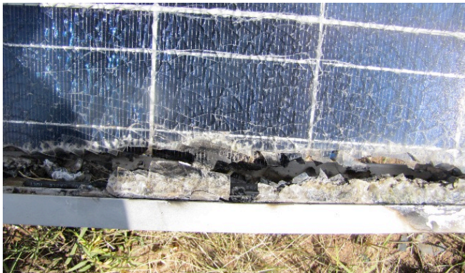
Fig. 2. Example of problem probably caused apparently by DC arcing between the frame and cells because the cells were too close to the frame to withstand the DC voltage between them.
