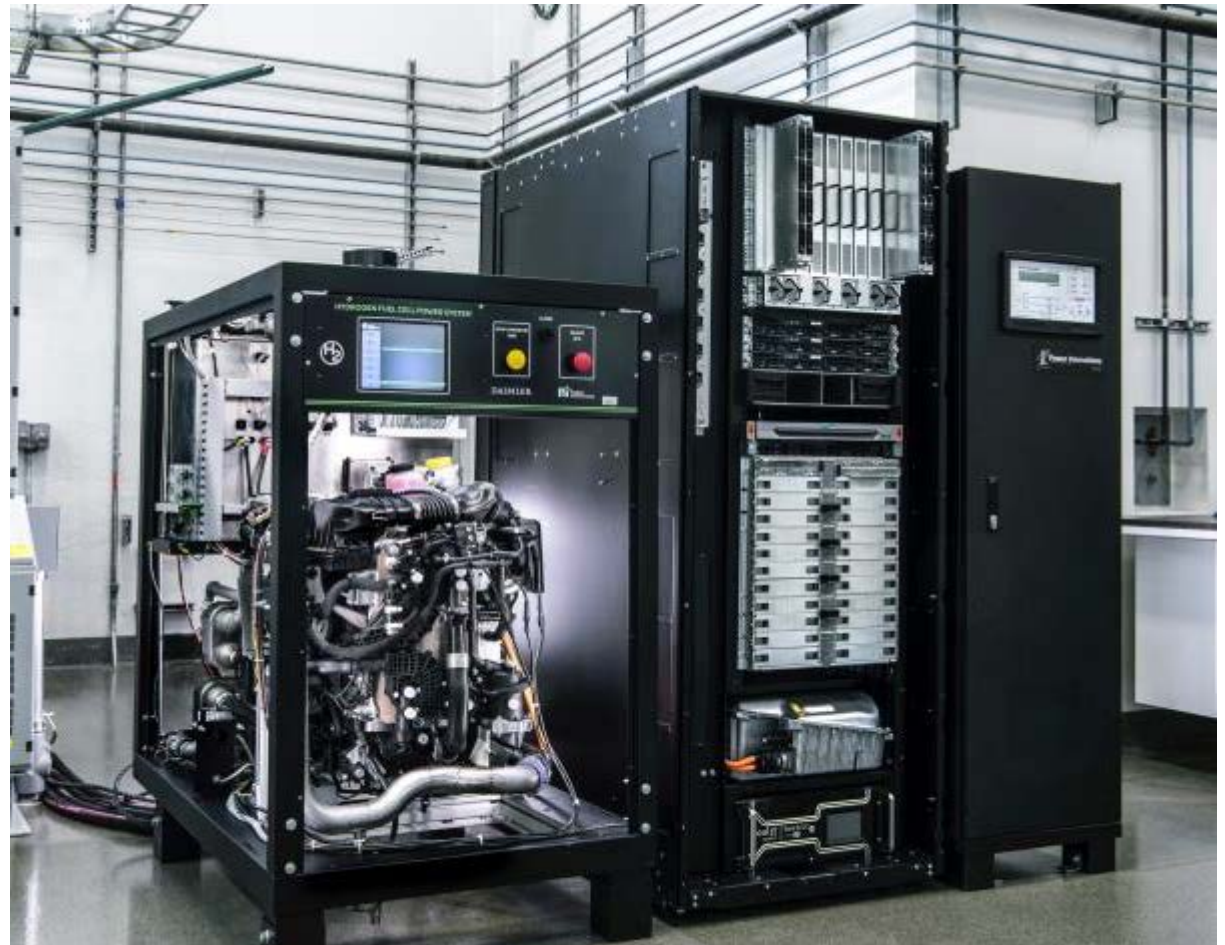
The integrated fuel cell and IT racks at NREL for initial shakedown this week.
