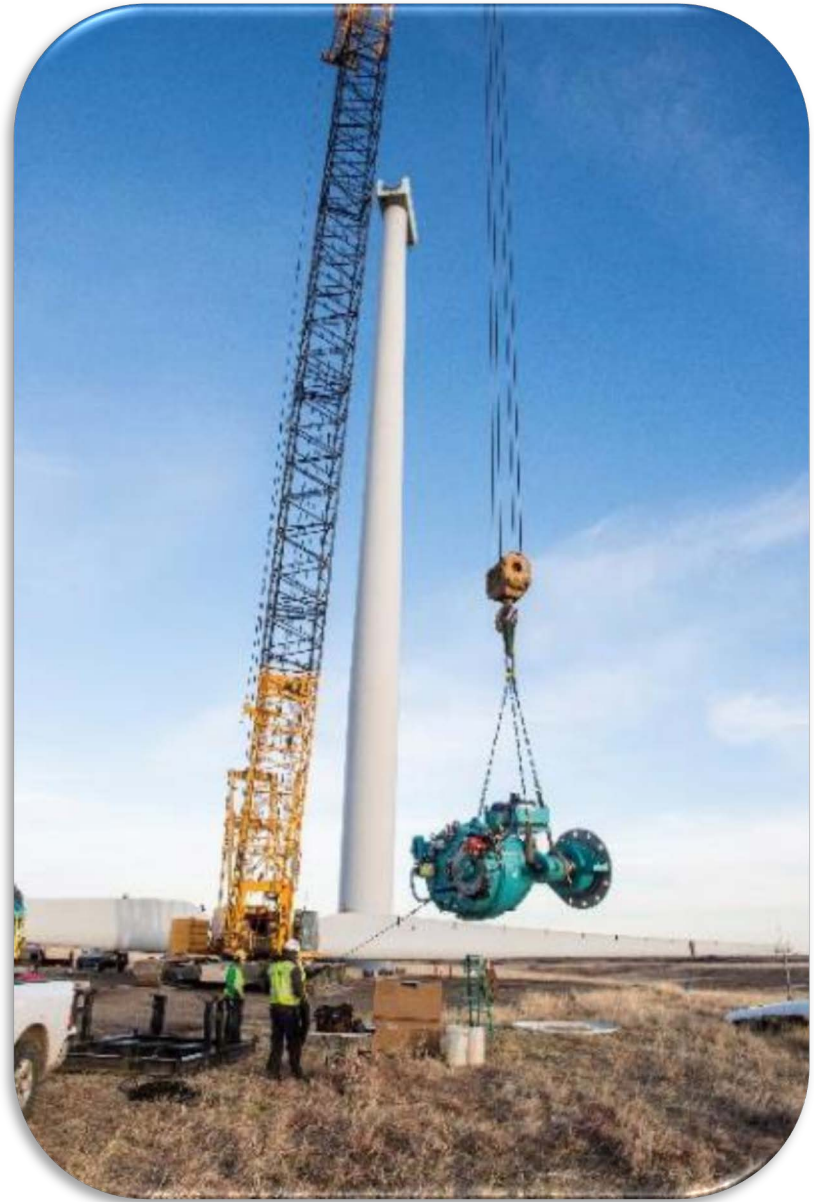
U.S. Department of Energy 1.5 rotor removal/gearbox swap at the National Wind Technology Center. Photo by Dennis Schroeder, NREL 49407
