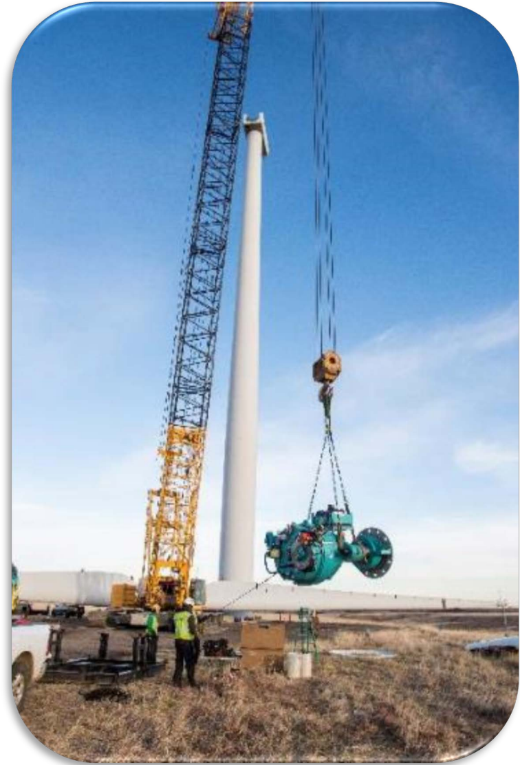
U.S. Department of Energy 1.5 rotor removal/gearbox swap at the National Wind Technology Center. Photo by Dennis Schroeder, NREL 49407
