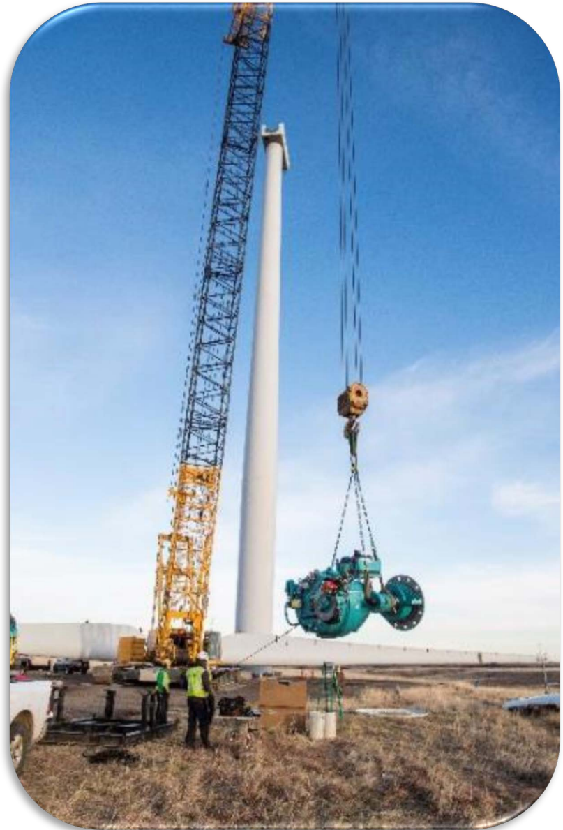
U.S. Department of Energy 1.5 rotor removal/gearbox swap at the National Wind Technology Center. Photo by Dennis Schroeder, NREL 49407
