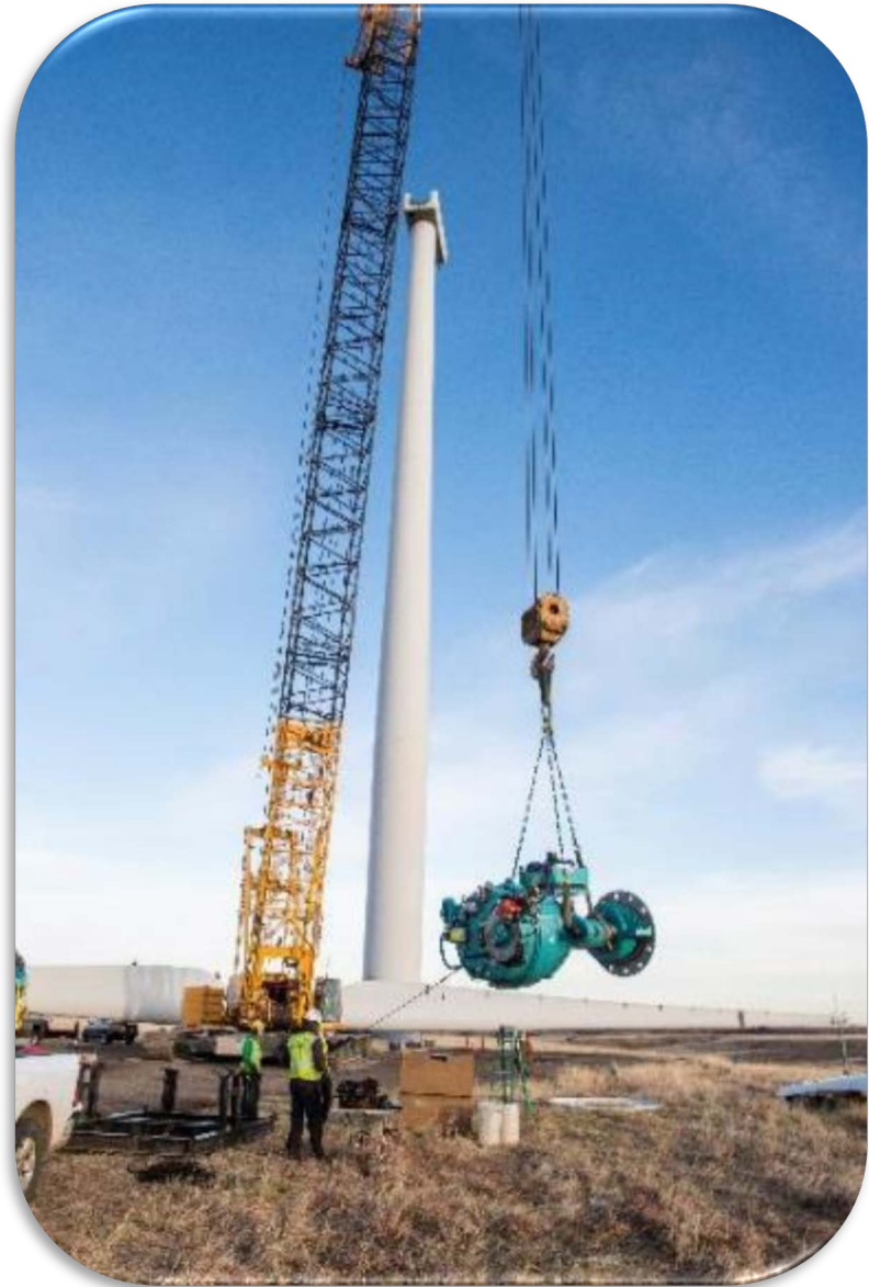
U.S. Department of Energy 1.5 rotor removal/gearbox swap at the National Wind Technology Center. Photo by Dennis Schroeder, NREL 49407
