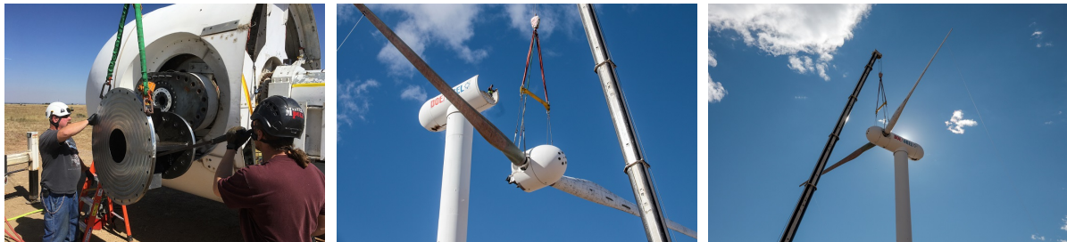
(a) NWTC technicians install one of the blade adapters to the CART2 hub.
