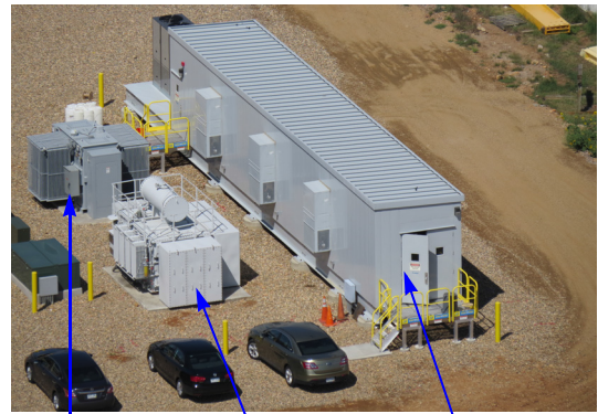
Fig. 2. 13.8 kV, 7 MVA grid simulator called controllable grid interface (CGI) custom designed using ABB's medium voltage ACS6000 drive technology.
