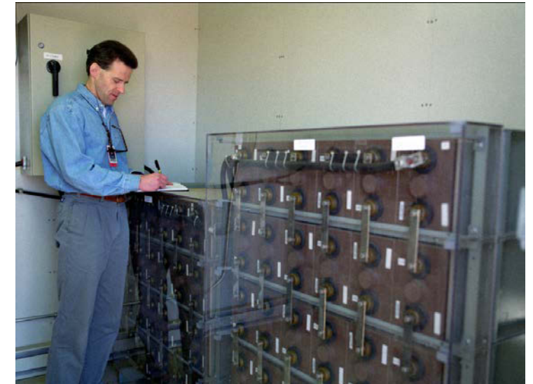
Battery Bank, NREL
