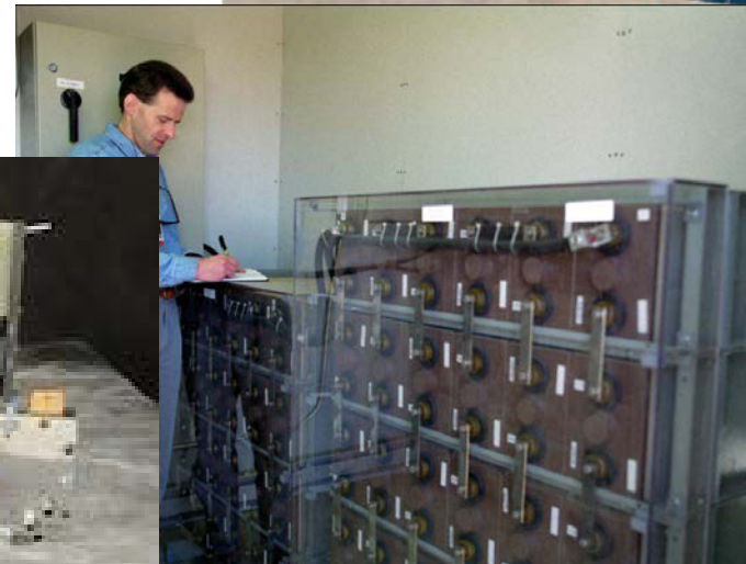
Battery Bank, Source: NREL
