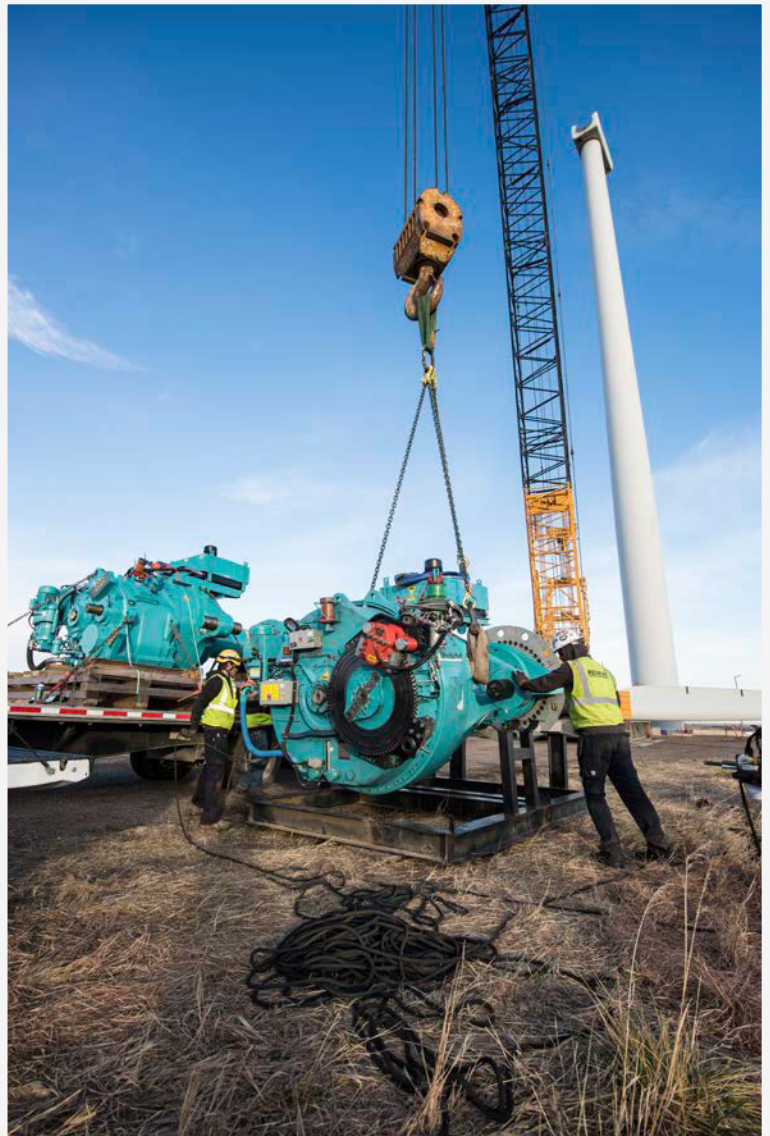
Workers swap out a wind turbine gearbox. Photo by Dennis Schroeder, NREL 49409
