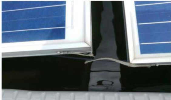
Mechanical Failure due to cyclic loading
