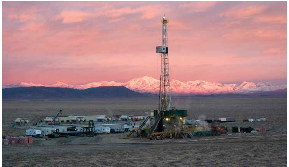
Drilling and power-plant construction at the Blue Mountain geothermal field in Nevada. Photo credit: John Casteel
