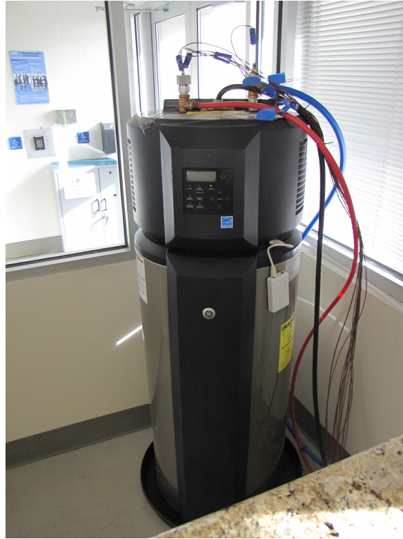
Figure 3. Residential water heaters are a flexible load that can provide a range of grid services—including load shifting and frequency regulation—without impacting occupants. This GE heat pump water heater is shown being tested at NREL’s Advanced Home Energy Management Laboratory. Image courtesy of NREL.
