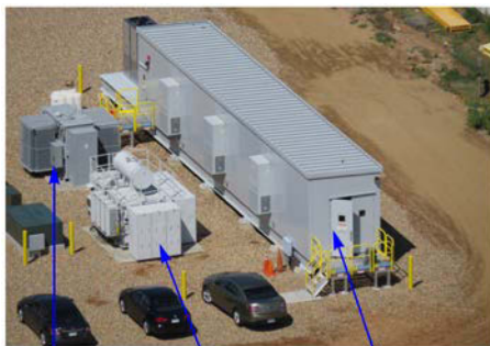
Grid-side transformer Output transformer ARU + 4 NP-VSC in parallel
