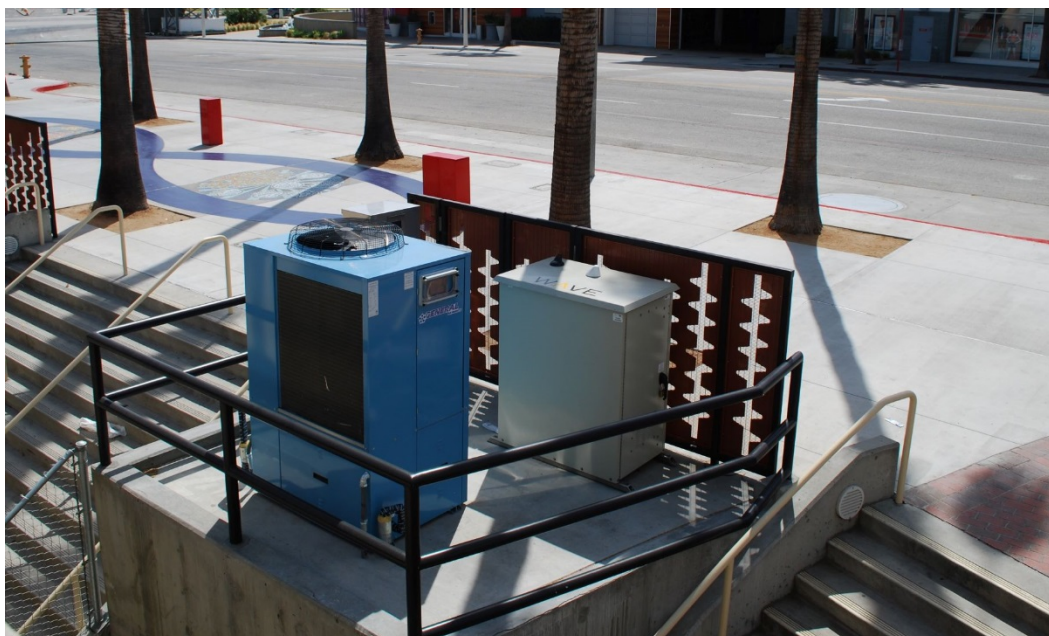
Figure 6. WAVE inductive charging station installed at the Long Beach Convention Center
