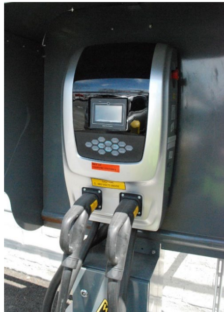
Figure 5. One of LBT's 10 chargers installed at the depot
