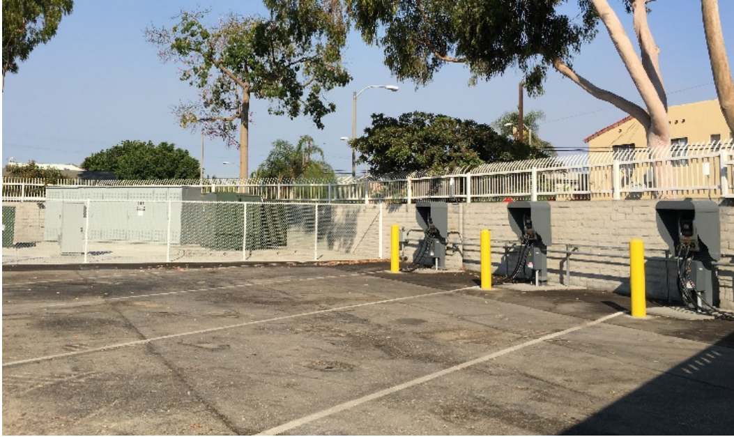
Figure 4. Row of BEB parking with chargers at the depot
