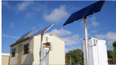
Utility Grid Connected
