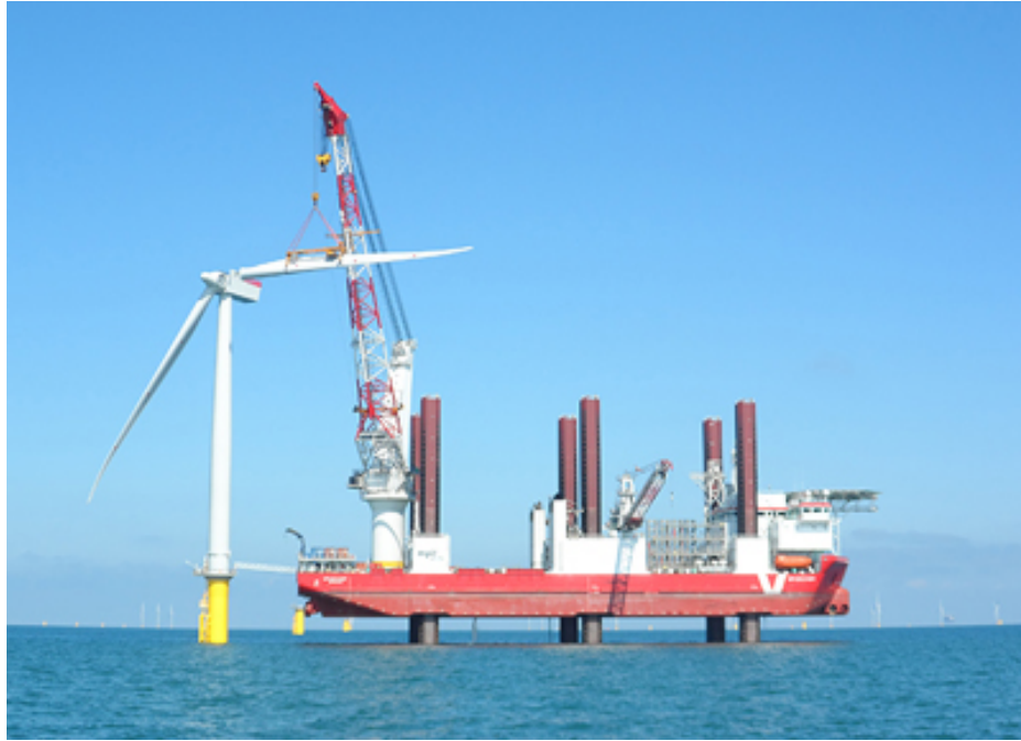
Figure 6. WTIV installing a blade at an offshore wind power plant. Photo from Siemens AG, NREL 27858
