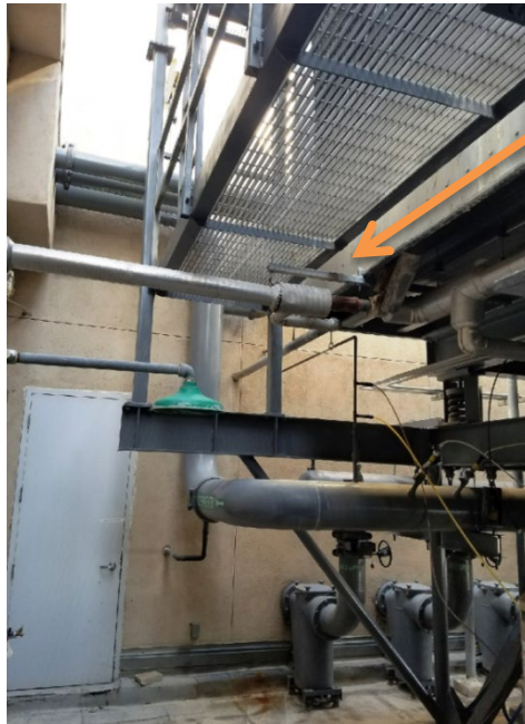
Figure 8. Cooling tower makeup flow meter location (Credit: Gregg Tomberlin, NREL)
