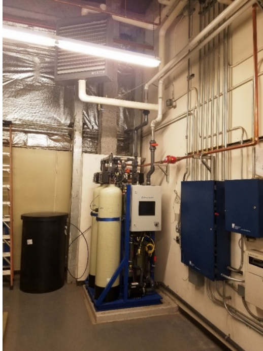
Figure 2. Aqualogix Lite Skid Location (Credit: Gregg Tomberlin, NREL)
