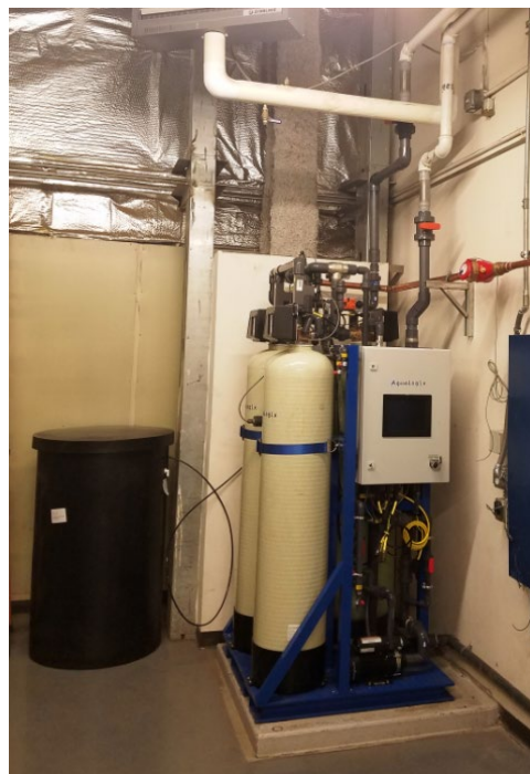
Figure 1. – AWT System at Lloyd D. George Courthouse
