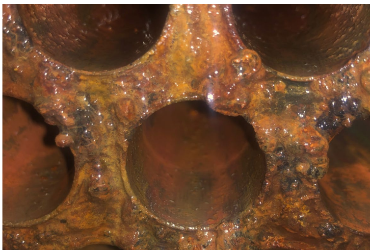
Figure 15. Condenser tubes after AWT testing (Credit: Jacob Lewis, GSA)
