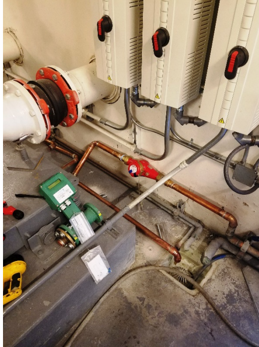
Figure 7. Cooling Tower Blowdown Meter and Piping (Credit: Gregg Tomberlin, NREL)
