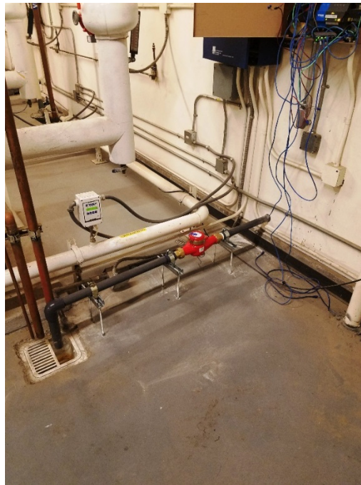
Figure 3 – Aqualogix Lite Blowdown Location (Credit: Gregg Tomberlin, NREL)
