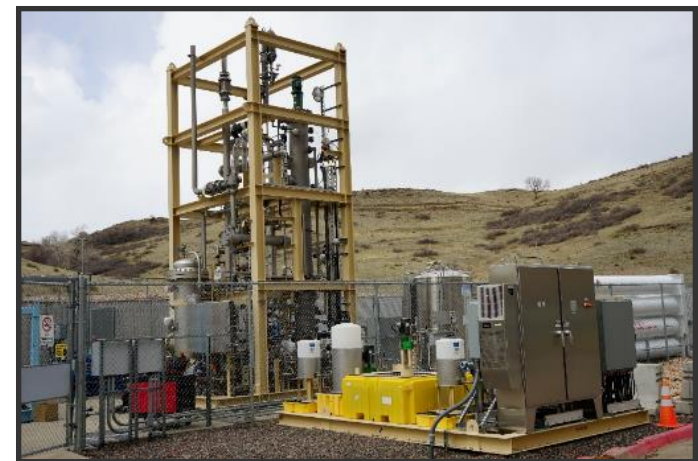
Biomethanation reactor (NREL)
