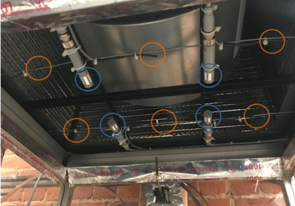
Figure 48. Six thermistors and four TRH sensors were installed to measure properties of the air entering the AHU (location 8 in Figure 47)
