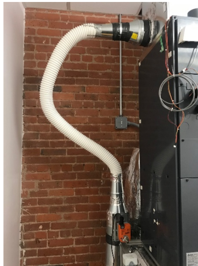
Figure 21. Tempering air for frost prevention drawn from AHU supply plenum
