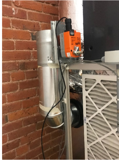
Figure 20. The tempering damper allowed room air to mix with outdoor air before passing through the core
