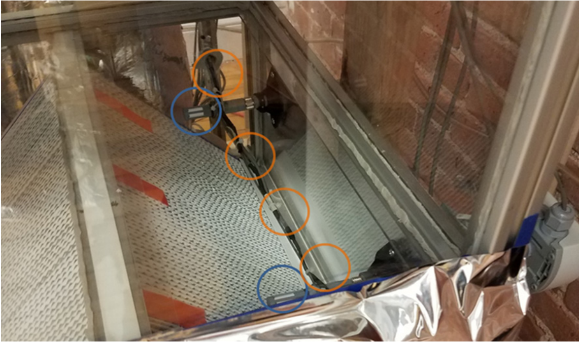
Figure 49. Four thermistors and two TRH sensors were installed in each quadrant where air left the ERV core
