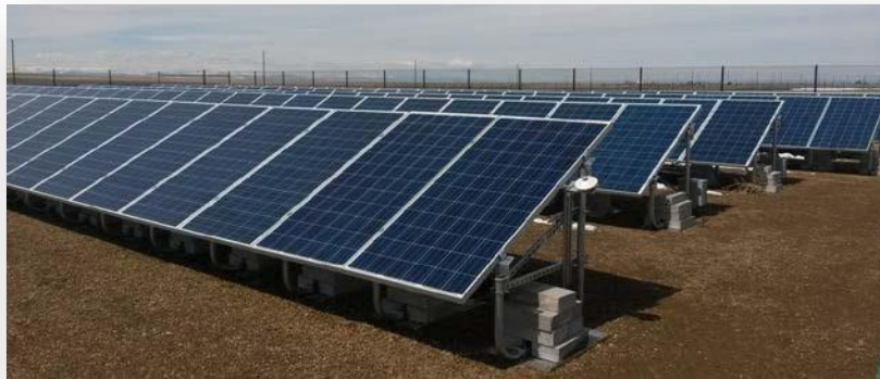
Figure 1: Maxim deployment at the NREL Solar TAC site
