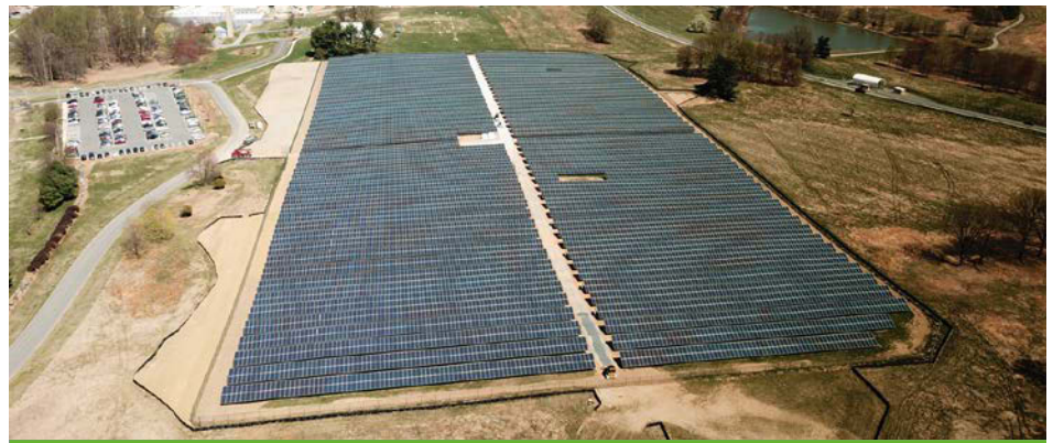
A nearly 15,000-panel solar PV array was installed under an ESPC ESA at the U.S. Department of Commerce's National Institute of Standards and Technology (NIST) in Gaithersburg, Maryland. The installation will be privately owned for the 20-year ESPC ESA term for tax incentive purposes and NIST will purchase the electricity produced. The array is predicted to save NIST a minimum of $3.5 million in its first 20 years of operation. Photo courtesy of NIST.
