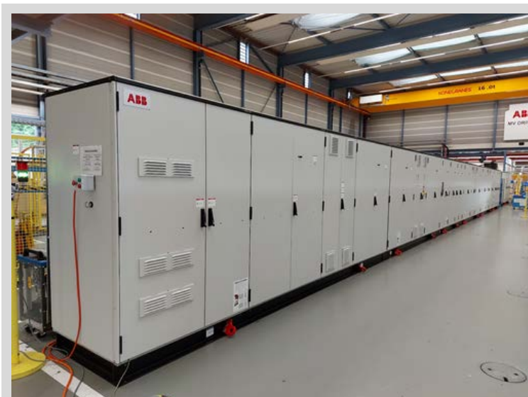
This converter assembly is a central component of the second controllable grid interface (CGI-2) at the Flatirons Campus. When complete, the CGI-2 will help the U.S. electrical grid evolve by allowing a greater contribution from variable power generators, increased levels of energy storage, and smarter grid devices. Photo courtesy of ABB Group
