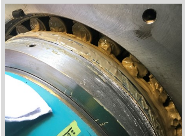
Grease is often used as a lubricant for rolling bearings to alleviate friction and wear. Over time, main bearing failures can still occur, which can increase maintenance costs and decrease wind power plant productivity. Photo by Photo by Mark Dunn, SKF
