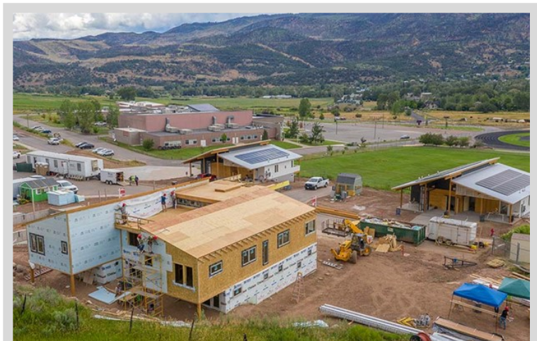
The Basalt Vista housing project, a collaboration between NREL and Holy Cross Energy, demonstrates the real-life applications of NREL's autonomous-energy-grid research. Photo by Scott Randall, NREL
