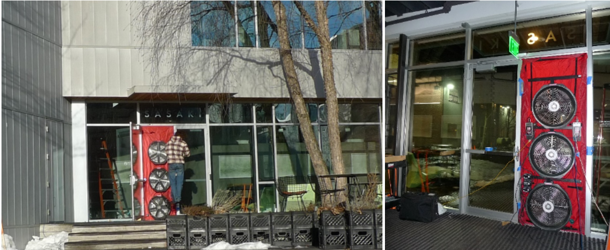
Figure 11. Blower door tests for commercial buildings can require much more equipment, which adds significantly to the setup and teardown time, as well as the complexity of performing the test itself.
