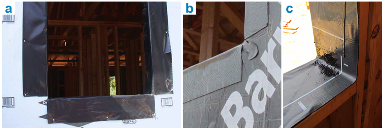
Figure 18. The corner of a roughed-out opening for a window in new residential construction is an example of the complex detailing required at interfaces to provide for air and water sealing. In (a), the air/moisture barrier has been wrapped around the window opening, but the corners have not been properly flashed, while in (b) and (c) the corners have been neatly detailed to ensure proper drainage around the window opening. The custom work required to accommodate each penetration through the facade creates a significant opportunity for errors and defects, which leads to variability in envelope performance from building to building.
