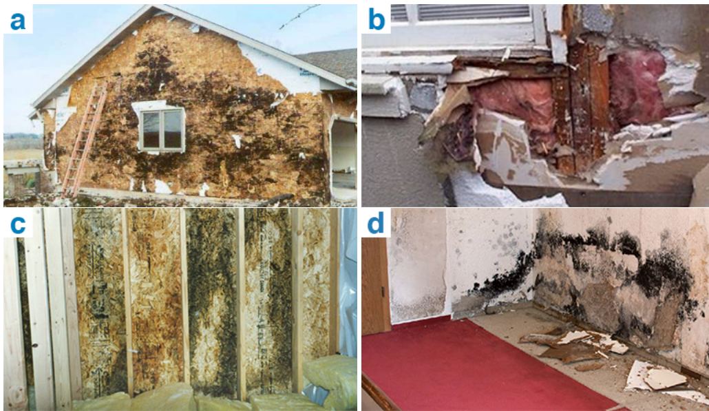
Figure 12. Examples of building envelope problems associated with extensive moisture intrusion. Photos (a) and (b) show the consequences of moisture intrusion and insufficient drying that has led to decay affecting multiple layers of the opaque envelope assembly. Photos (c) and (d) show the effect of moisture intrusion on the interior side of the opaque envelope.
