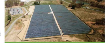
A nearly 15,000-panel solar PV array was installed under an ESPC ESA at the U.S. Department of Commerce's National Institute of Standards and Technology (NIST) in Gaithersburg, Maryland. The installation will be privately owned for the 20-year ESPC ESA term for tax incentive purposes and NIST will purchase the electricity produced. The array is predicted to save NIST a minimum of $3.5 million in its first 20 years of operation. Photo courtesy of NIST.
