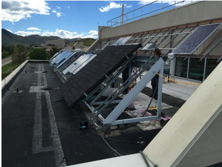
Fig. 1. Completed artificial roof surface ready for the installation of the Omnisole products.
