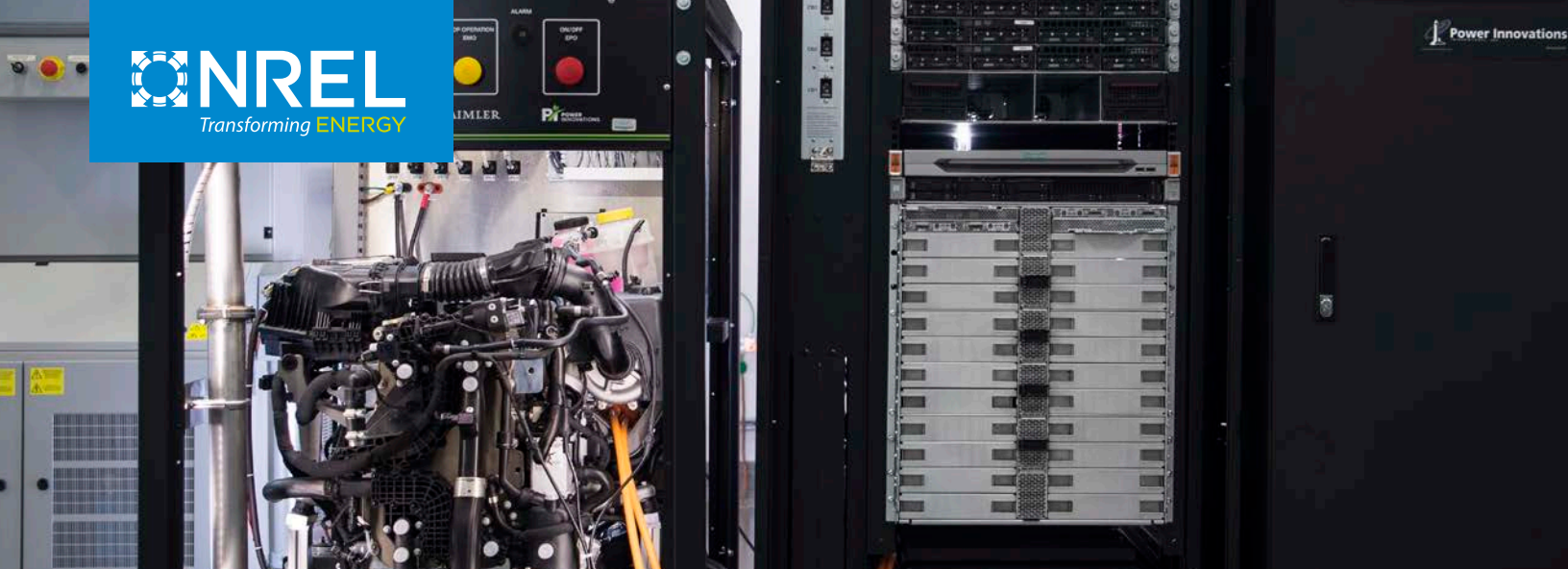
The Hydrogen Fuel Cell Power System, being tested in the Energy Systems Integration Lab in the ESIF before it is moved into the High Performance Computing Data Center. Photo by Dennis Schroeder, NREL 48948.
