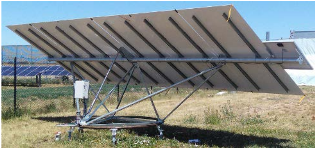
Figure 12. Rear view of the SunRing heliostat at the Solar Technology Acceleration Center, showing the pilings, base, drives, and mirror support structure
