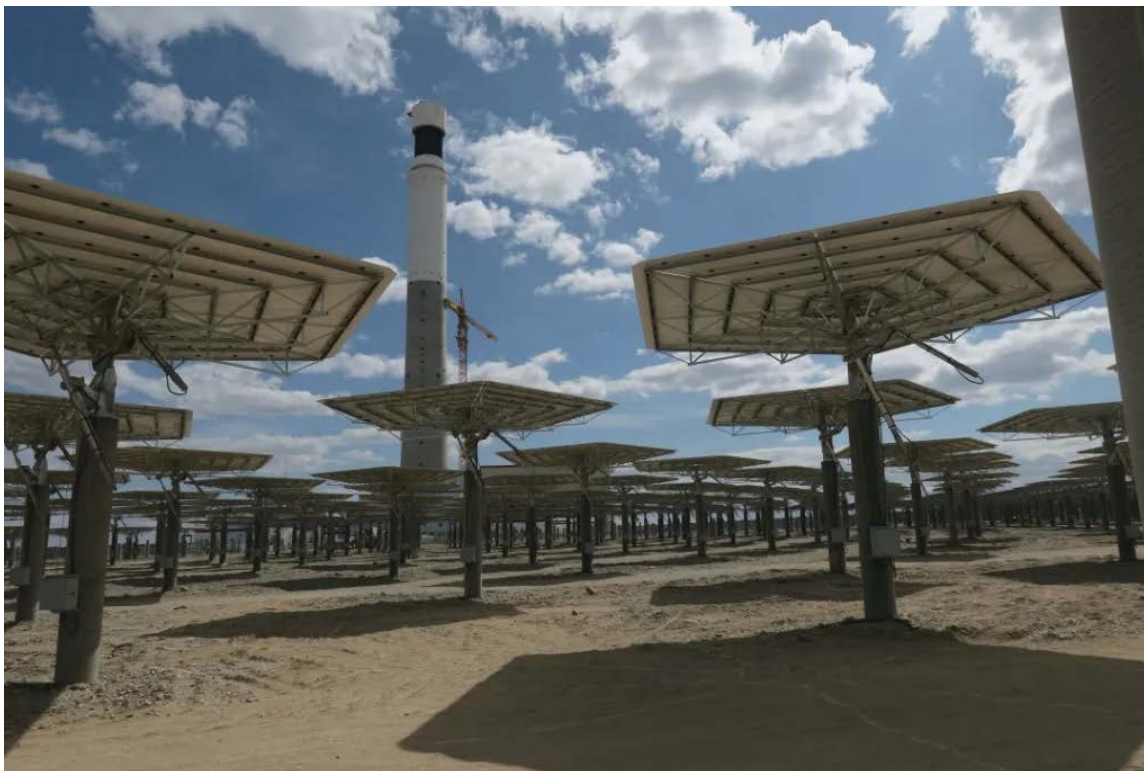
Figure 3. Stellio heliostat field for the 50- MW_e molten salt solar tower project at Hami
