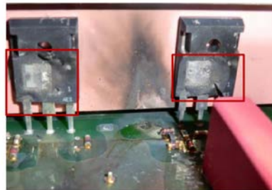
IGBT burnout failure
