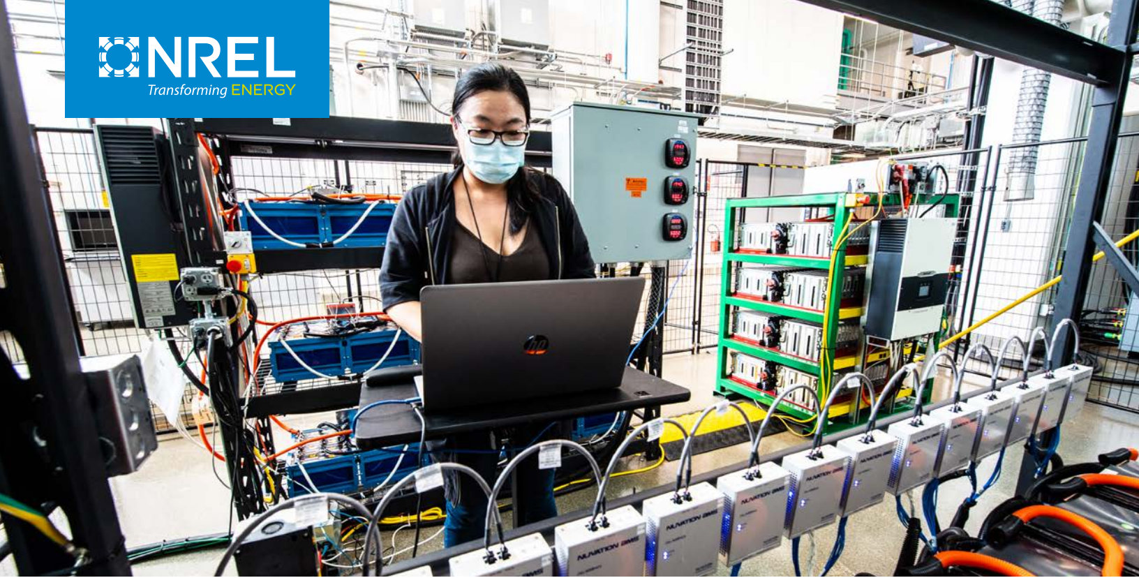
NREL researcher Ying Shi works on NREL's Centrica hybrid battery energy storage system, which includes second-life batteries. Photo by Dennis Schroeder, NREL 62826
