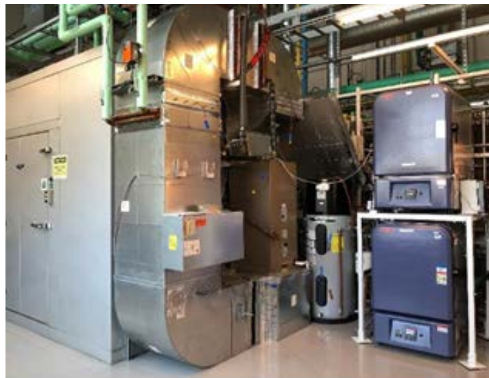
Figure 2. Hardware installed in the SPL for HIL experiment. The grey chamber on the left contains the condenser with the air handler and duct loop next to it. The top blue chamber on the right houses the thermostat.
