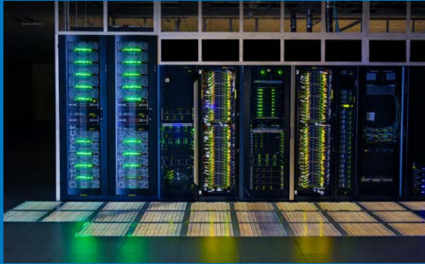
High Performance Computing Data Center at the National Renewable Energy Laboratory. (Photo by Dennis Schroeder / NREL24358 )
