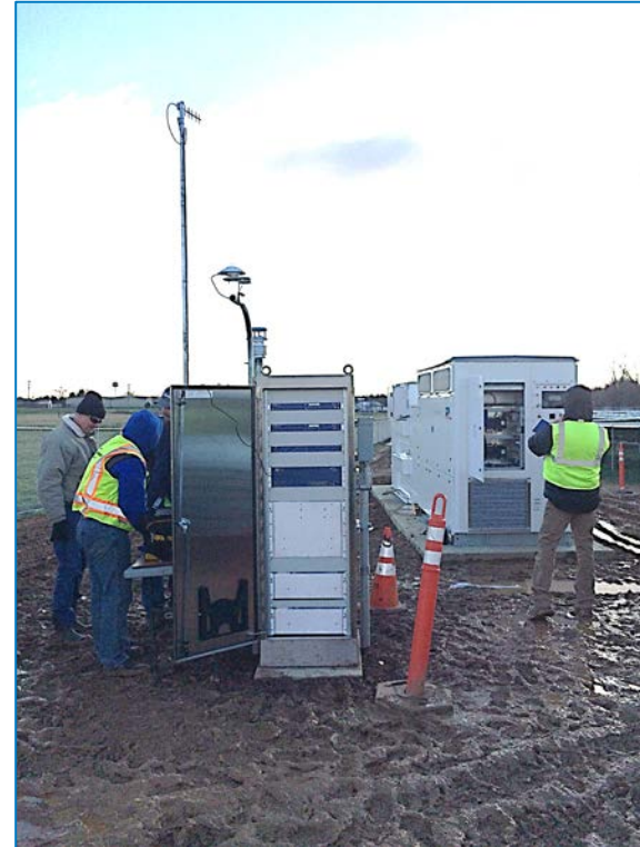
PV System Control and Data Acquisition System including Radio Communications (Photo by Andy Walker, NREL)
