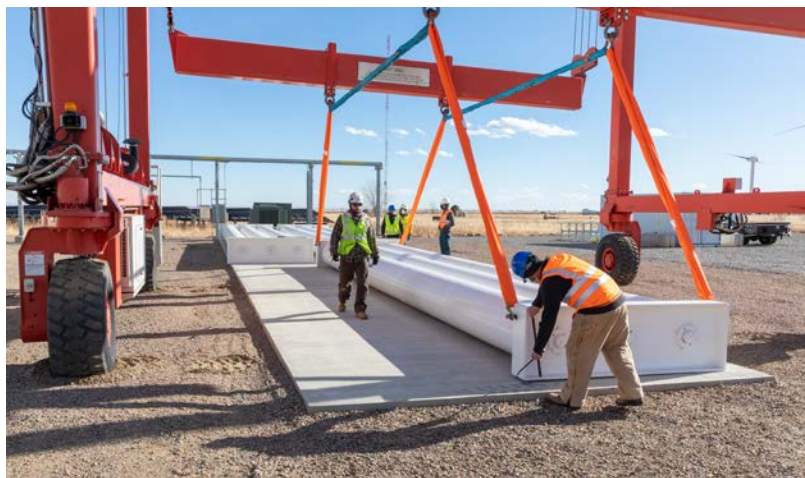
Installing hydrogen storage at ARIES. Photo by Werner Slocum, NREL
