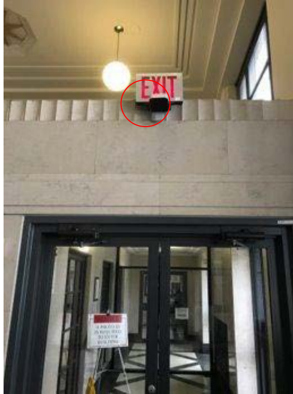
Figure 3: Stereoscopic occupancy counter at Terminal Annex Federal Building. Photo by Joshua Banis, GSA
