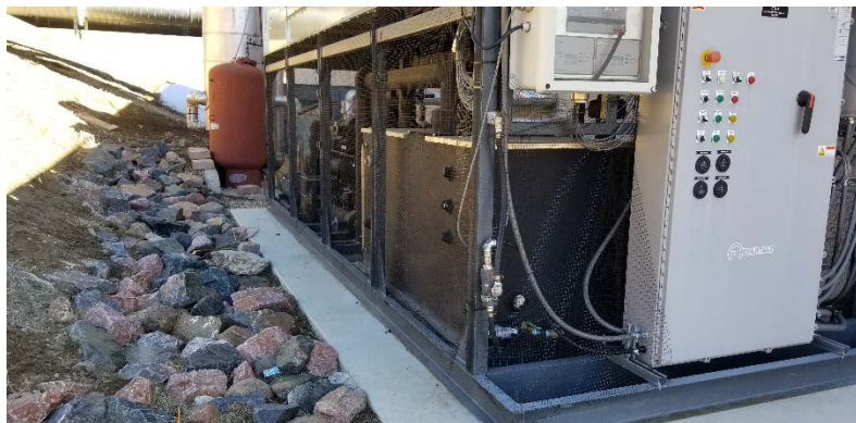
Figure C-2. Noncombustible zones should also extend 5 feet from equipment that may ignite
