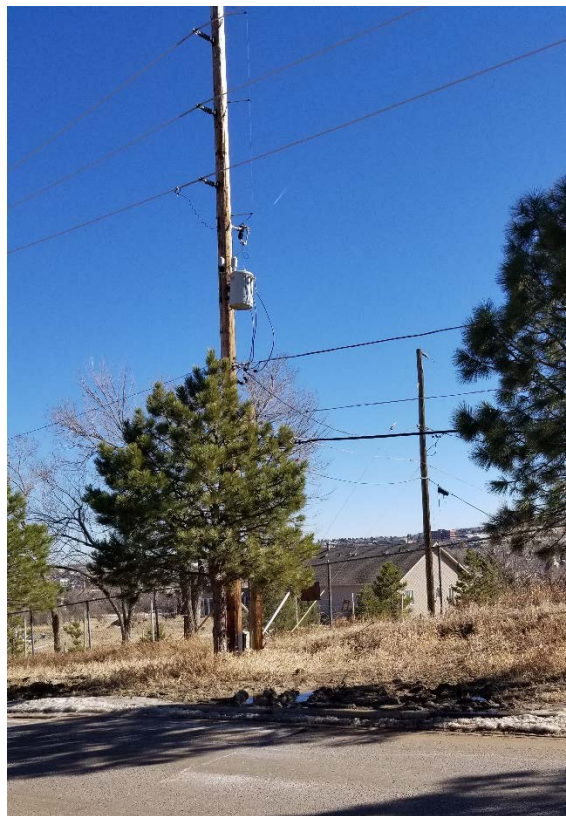
Figure C-26. While the tree is not tall enough to merit trimming from the top, the grass should be mowed at the base of this pole with a transformer
