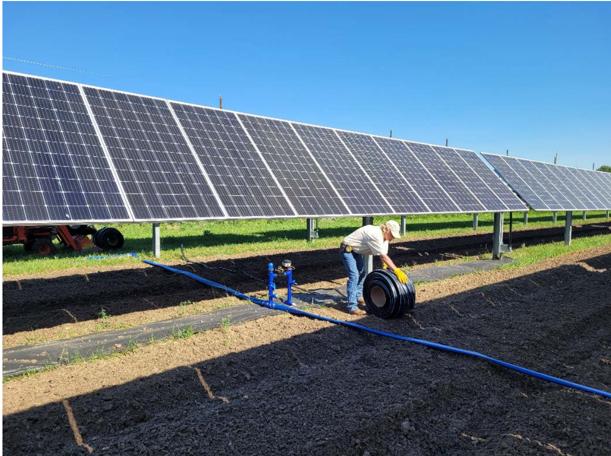
Figure 20. Irrigation equipment and infrastructure at an InSPIRE agrivoltaics site that can affect farm equipment access.
