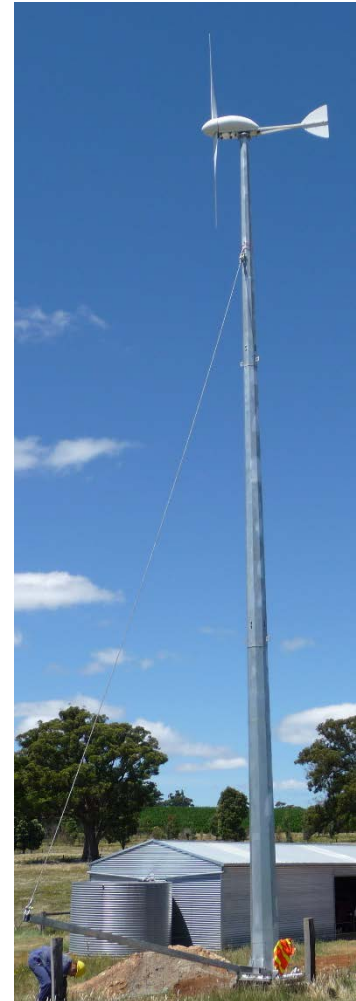
Figure 4. The Aerogenesis 5-kW SWT on its monopile tower
